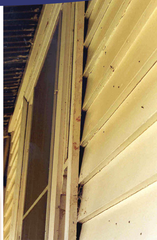
A colony of bats roosted behind the window frame, leaving the tell-tale sign of droppings on the wall. Photo: Lindy Lumsden
